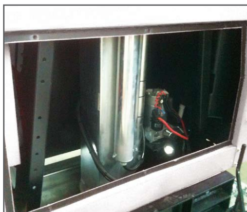
▲ Hydraulic pump maintenance compartment
