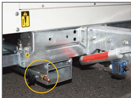
▲ Metal earthing bar
